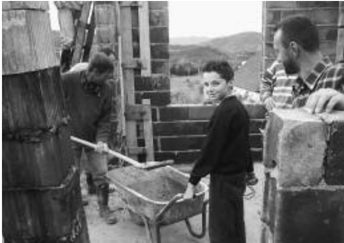
Fourteen year old Ahmo Habibovic, enthusiastically lends a hand on construction of new house for his six family members, driven from Srebrenica and re-united after their father was released from five months of torture in a concentration camp.
